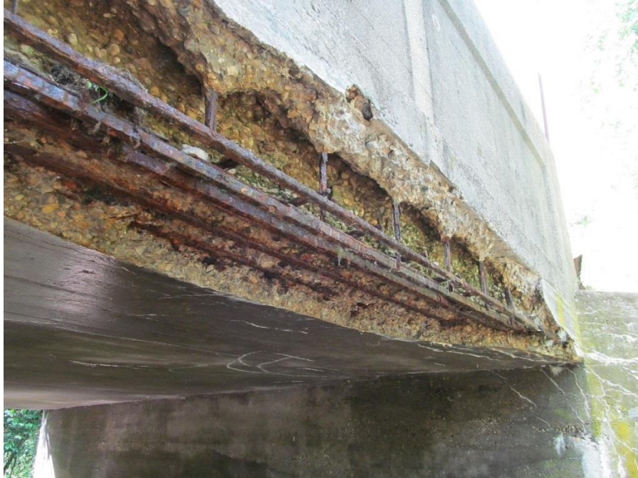
Figure 3. Spalled concrete and exposed reinforcing bars along east edge of deck soffit.
