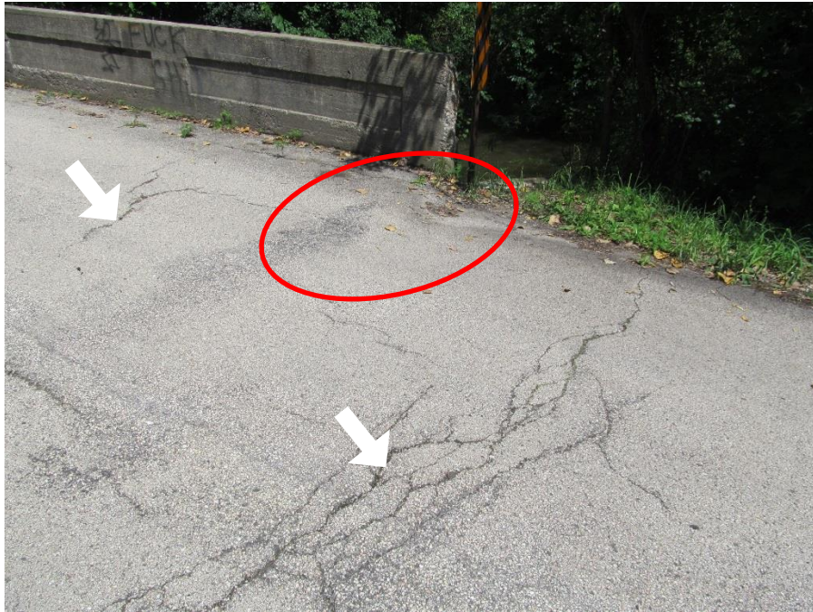
Figure 5. Settlement of approach pavement at the southeast corner of the bridge deck (arrow) and transverse cracking of the asphalt pavement (arrows).
