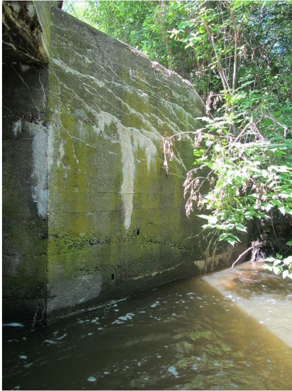
Figure 7. Freeze/thaw damage at the top of the northeast wingwall highlighted by cracking with efflorescence.
