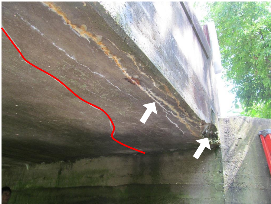
Figure 4. Spalled concrete and efflorescence (arrows) at southwest corner of the deck soffit (red line shows extent of delaminated concrete).
